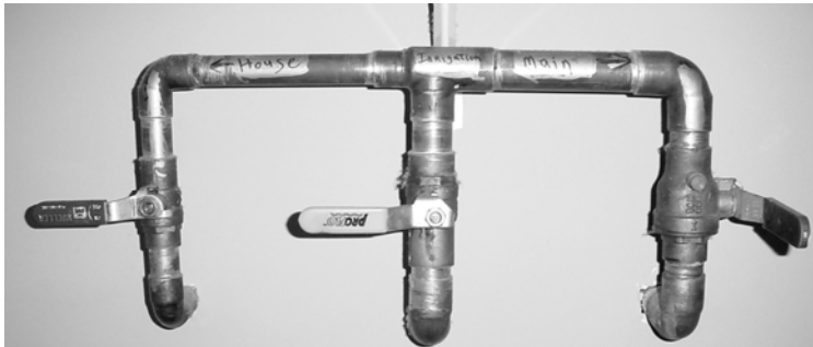
Typical ball valve arrangement, all in the closed position.
